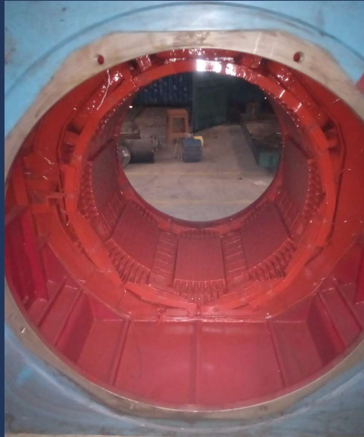
DC motor 1250 kw PT. SANXIONG STEEL
